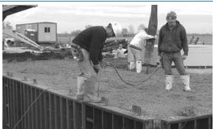
Wind Power: Contractors pour the foundations of a large wind turbine at Erie CUSD 1 on December 29. To learn more, visit: http://www.erie1.info/ .
