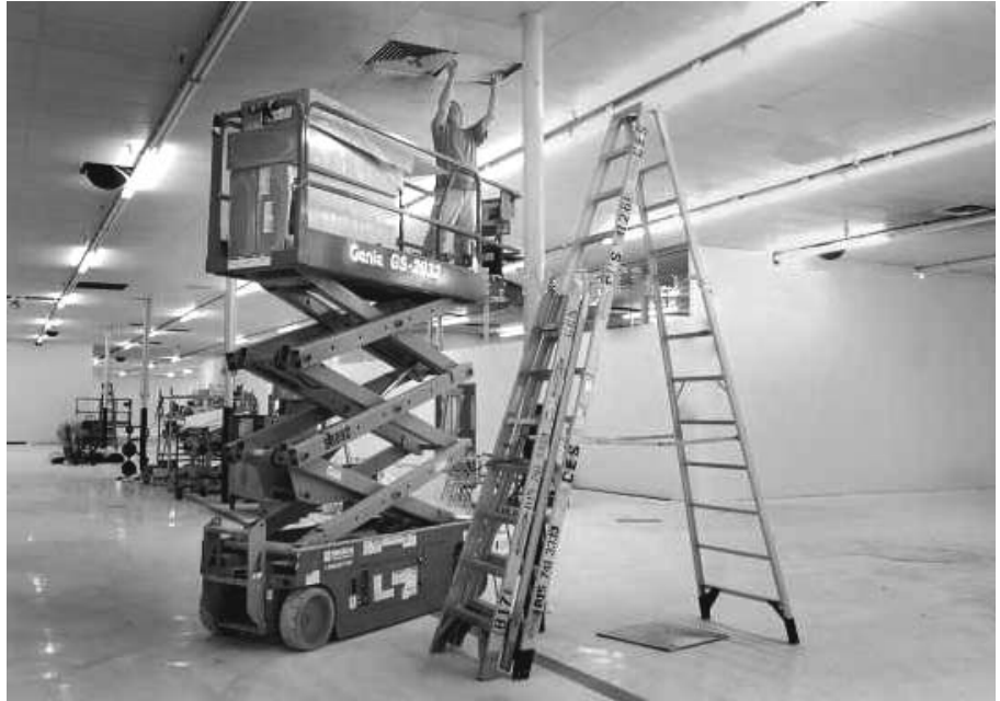
A workman replaces a ceiling tile in an old Wal-Mart building as remodeling is finished up in preparation for Central School students to attend classes there this fall at 2901 N. Columbus Street, Ottawa.
