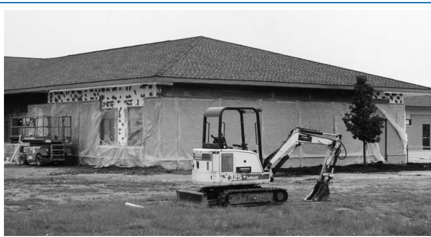
Construction is nearing completion on the addition to IASB's Springfield headquarters, which is designed to boost delivery of services by adding space to the warehouse at the back of the building.
